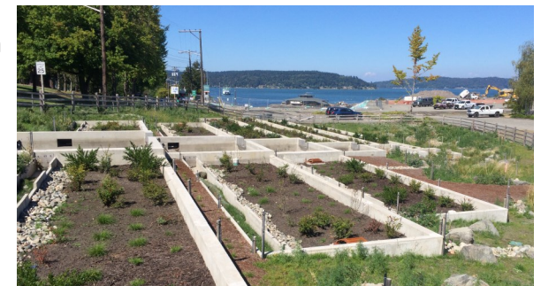
Point Defiance treatment facility.
