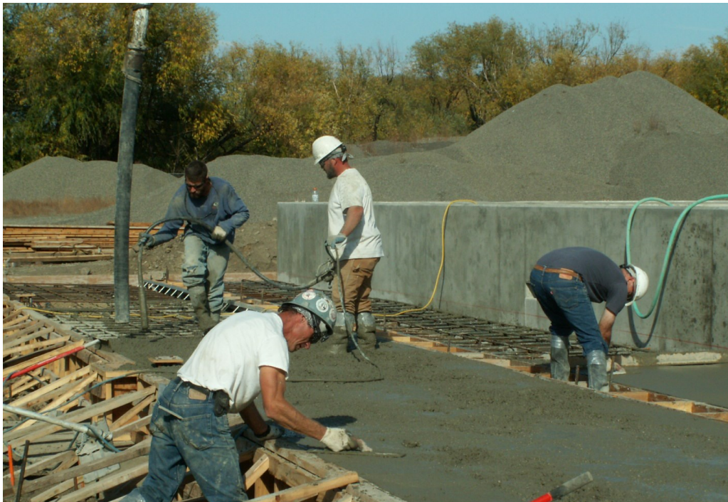
Ellensburg Decant facility helps keep pollution out of stormwater.
