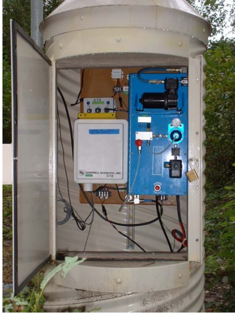
Figure 4: Campbell Scientific Data Collection Platform (CSI DCP) with the blue Hydrological Services bubbler system on the right, and white enclosure containing CSI electronics components on the left. (Photo by Washington Dept. of Ecology)
