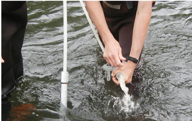
Figure 3 – Bilge pump development of a steel piezometer
