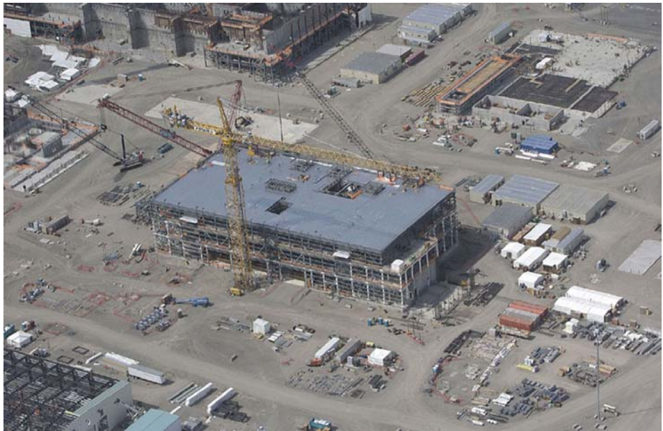
The Waste Treatment Plant is currently under construction at the Hanford Site. This aerial photograph shows the progress of the Low Activity Waste facility in June 2006.
