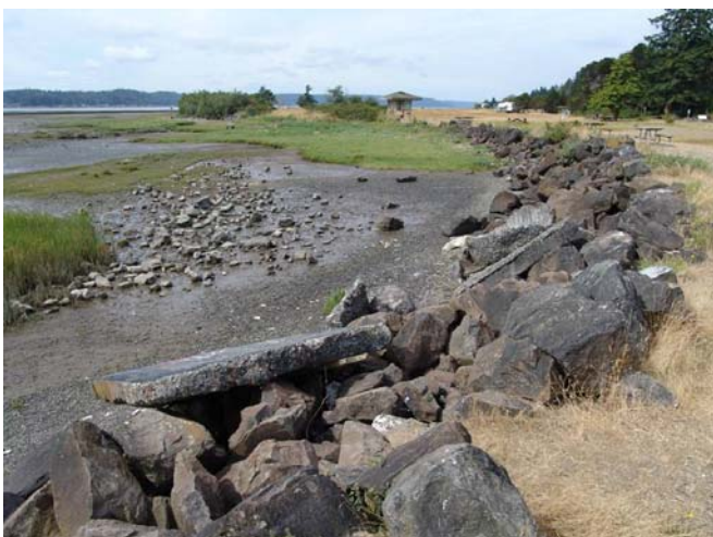
Big Mission Creek estuary at Belfair State Park before November 2006. Rock walls inhibit the natural functions of shorelands, estuaries, bays and river banks.
