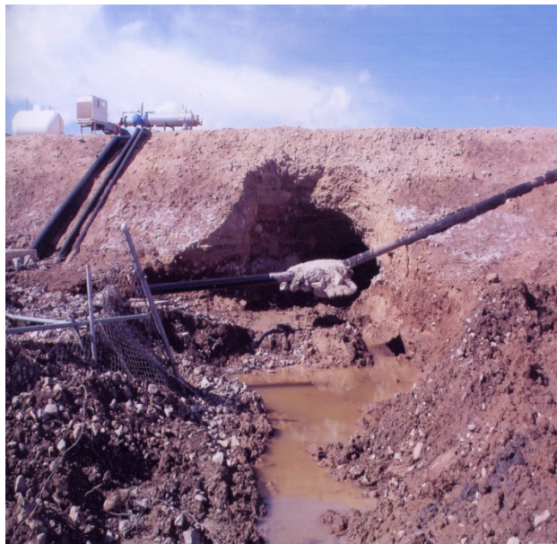
Kershaw Dam failure in Yakima County in April 2005.
